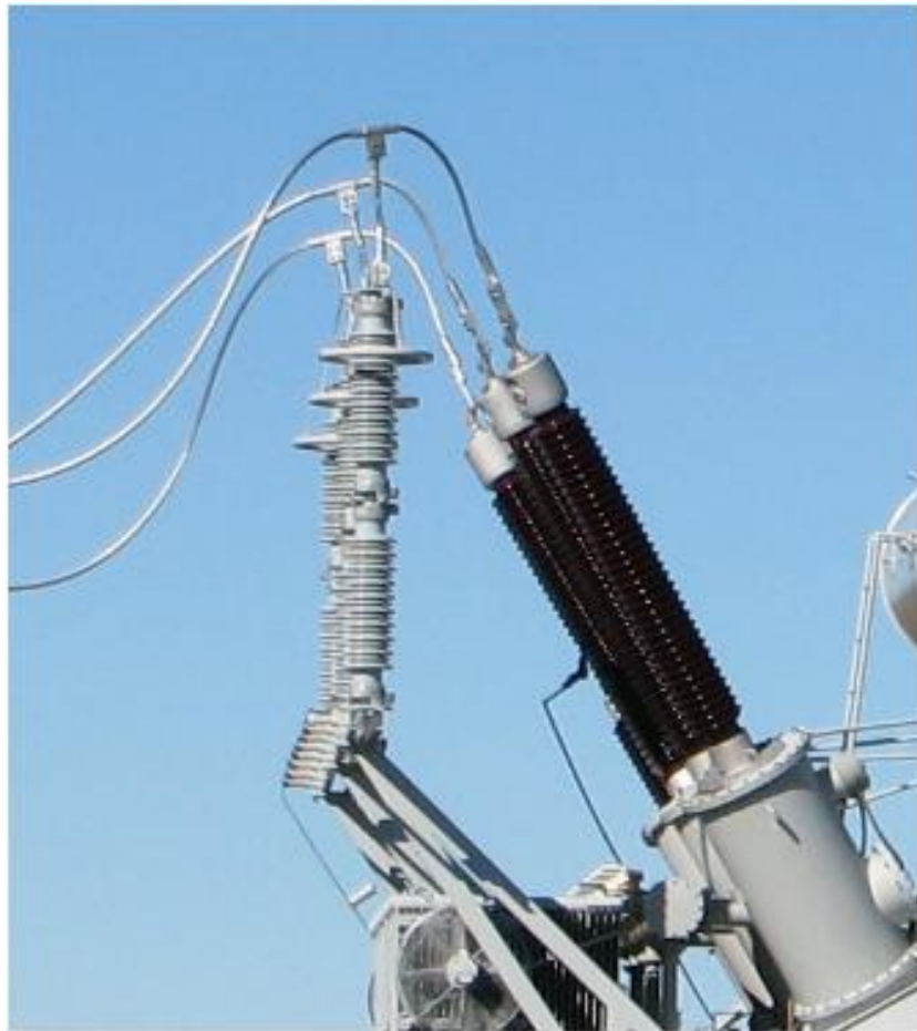
Figure 2 Arresters' with large diameter leads due to mechanical strength requirements
