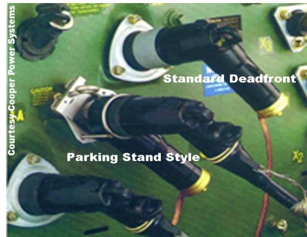
Figure 9 Underground Circuit with Deadfront Arrester one cable span from end point
