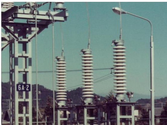
Figure 2 The first ZnO surge arrester (MOSA) in the world
