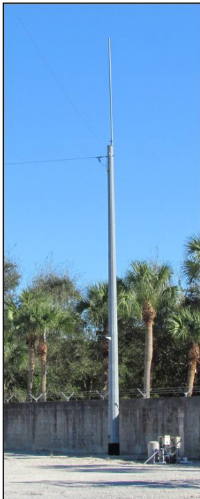
Figure 3 - Lightning Terminal in Substation
