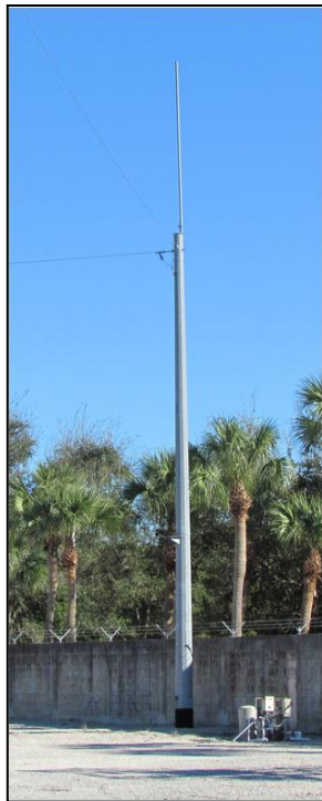
Figure 3 - Lightning Terminal in Substation
