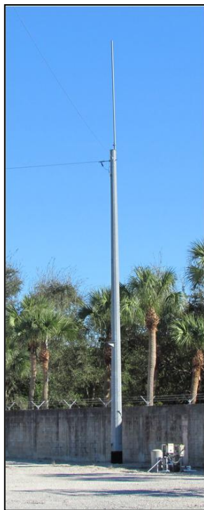
Figure 3 - Lightning Terminal in Substation
